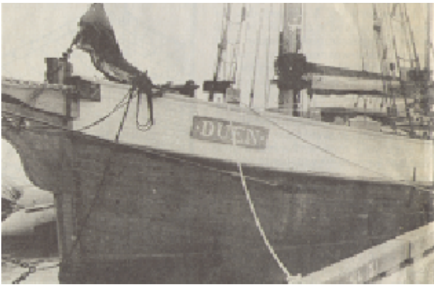
The wood trunnels fastening the Duen's lower hull planks are visible in this June 30 photo of the boat in Ketchikan
